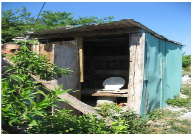
Picture 17: Condition of pit latrines that are being used by households
